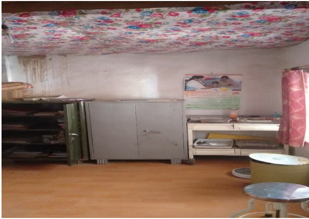
Room needs major repair
