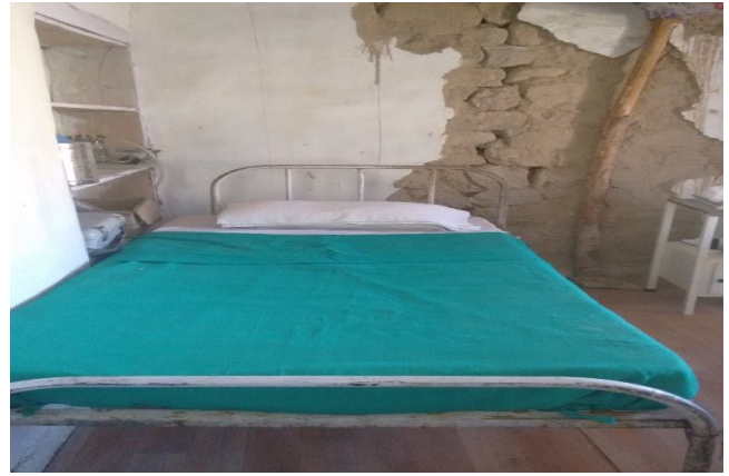
Clean bed but broken walls
